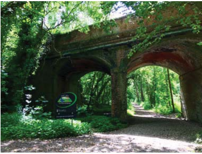
3 THE RIVER ANTON WAY ENDS WHERE IT MEETS THE TEST WAY UNDER A3057 ROAD BRIDGE
