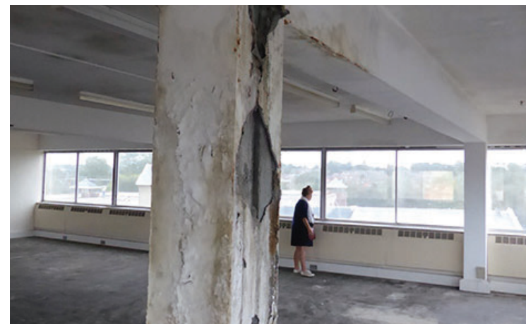
Poor quality office space above the centre
