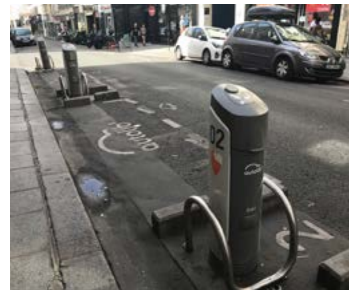
Efficient & unobtrusive charging banks / Paris
