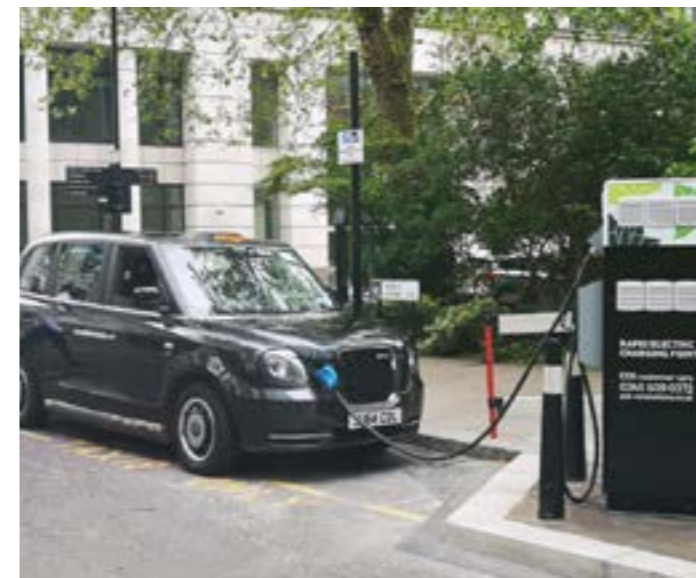
Free-standing rapid charging point / London
