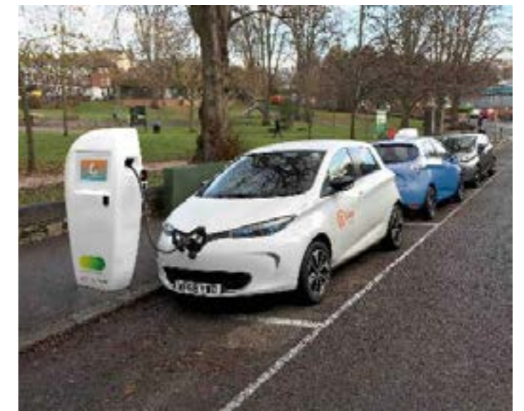
Unacceptable placement of chargers / Devon
