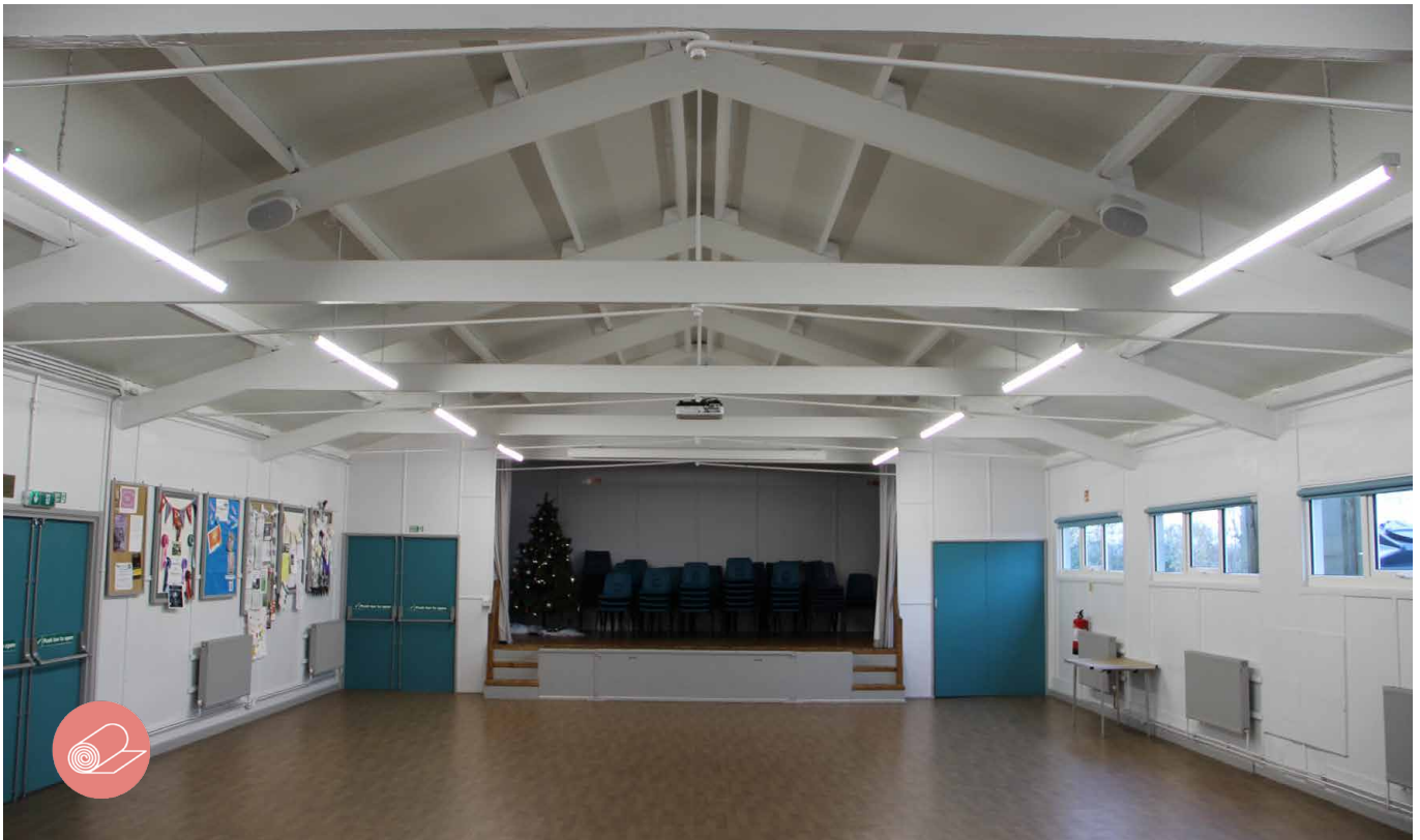
New low-energy LED lighting was installed and the hall decorated to give it a fresh and bright appearance
