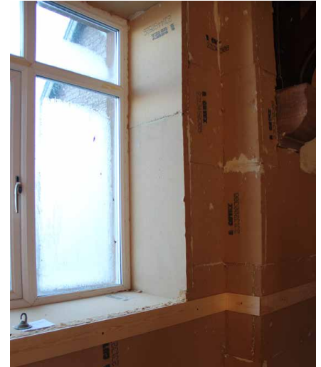
Wood-fibre board insulation fixed internally and turned into the reveals to meet the window frame at Skelton Toppin Memorial Hall.
