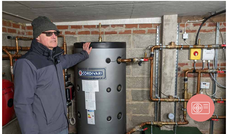
The internal part of the ground source heat pump is located in a semi-basement beneath the stage area
