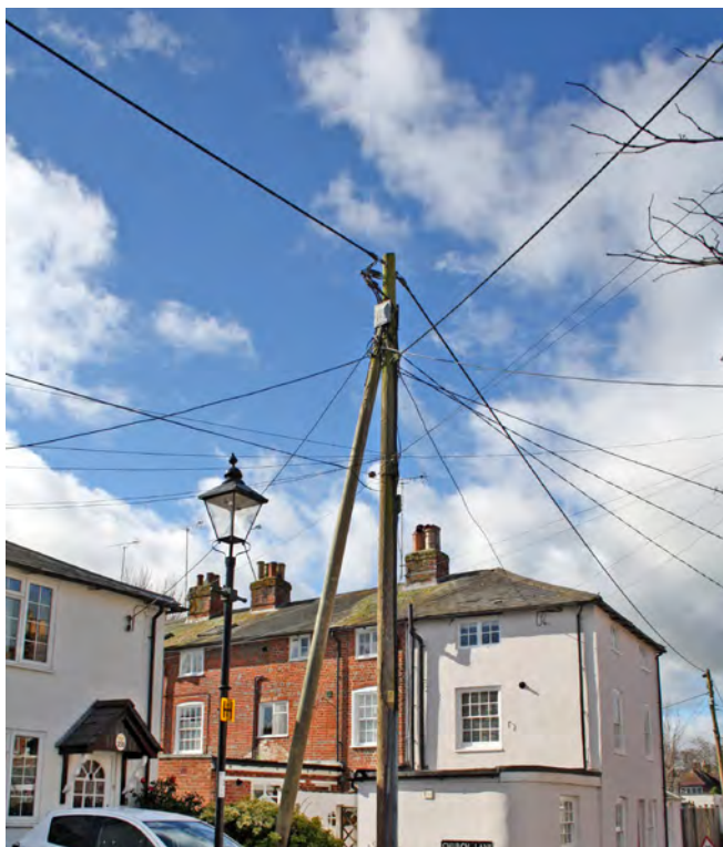
Overhead wires in Mill Lane
