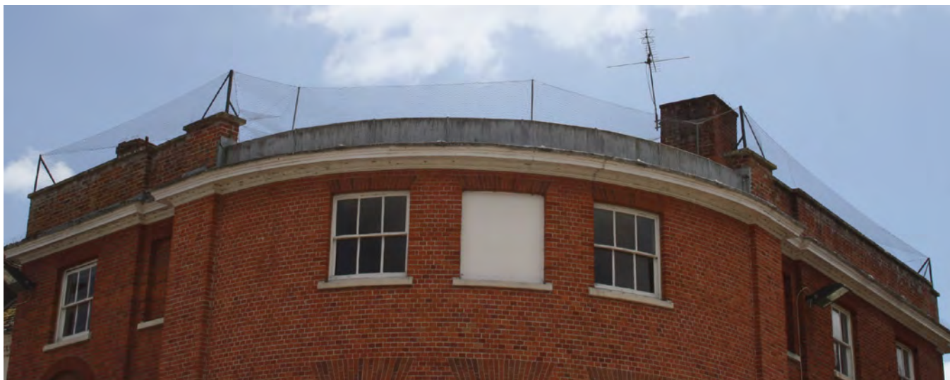
Example of visually prominent pigeon netting which detracts from the appearance of the Conservation Area
