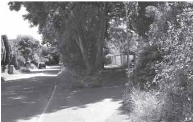
Raised pavement by Mountbatten School
