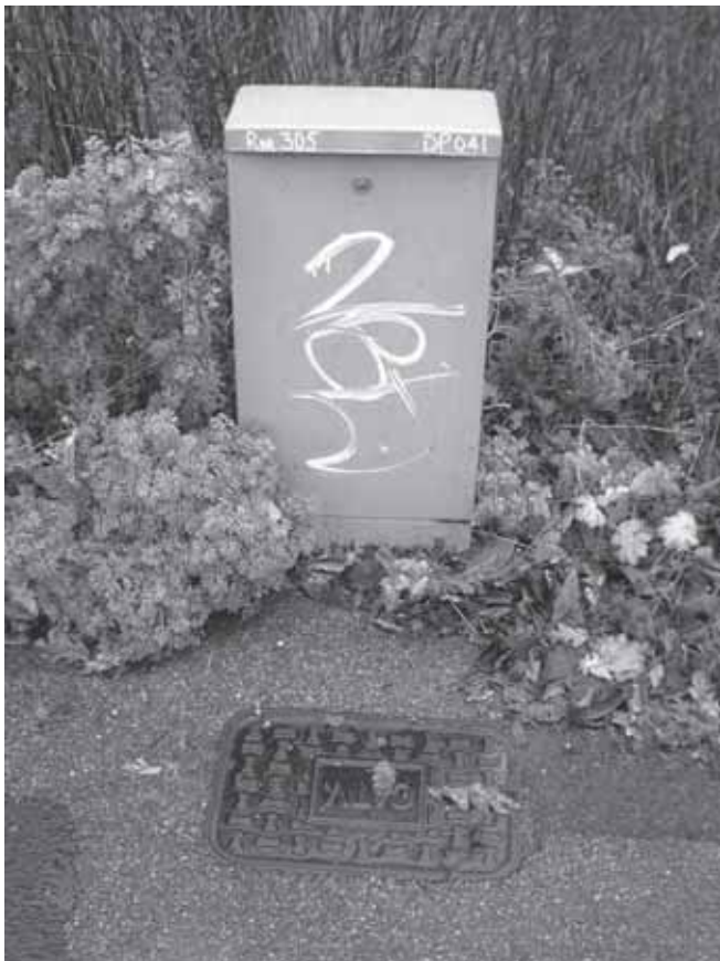
Junction box disfigured by graffiti
