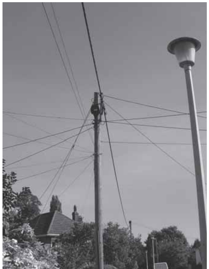
Overhead cables dominating the skyline
