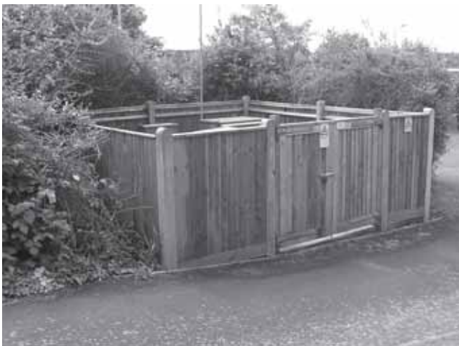
Substation road view, Woodley Lane
